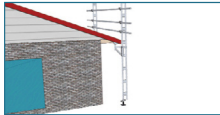
STEP 5 USING A LADDER, PLACE THE ALUMINIUM TUBE RAILS IN POSITION, THEN TIGHTEN EACH COUPLER
